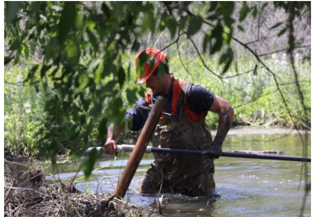
Figure 2f. A hole in the dam is created with a ramrod and then the explosive is seated in the hole created.
